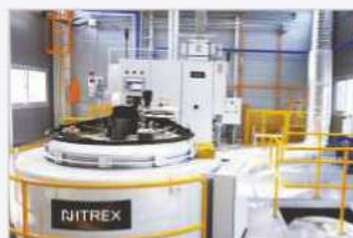
Gas Nitriding furnace
